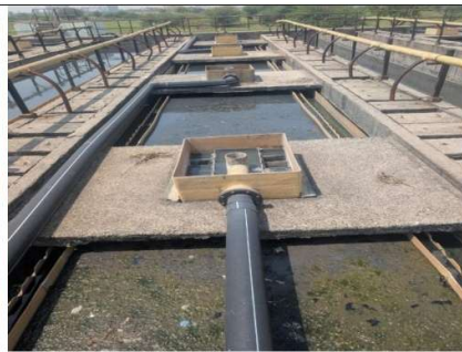
Division boxes on UASB
