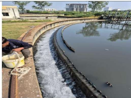
Secondary clarifier with broken baffle
