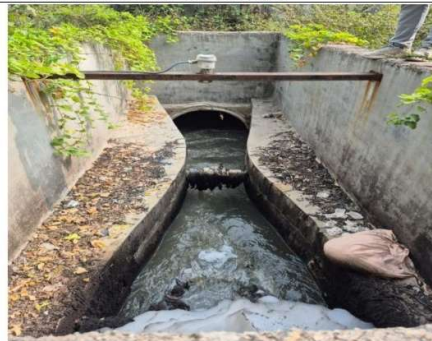
Parshall Flume covered with foam.
