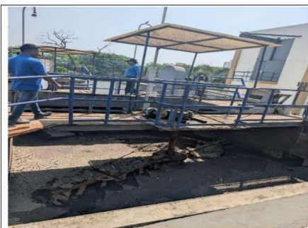
One of the grit chambers is defunct
