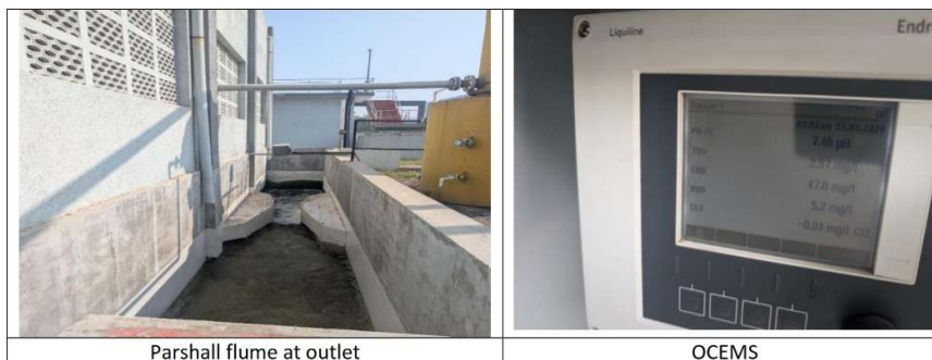
Parshall flume at outlet
