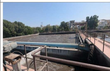
SBR in aeration mode
