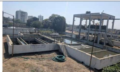
Tertiary treatment out of order
