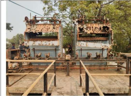
Both screen chamber is not in working condition
