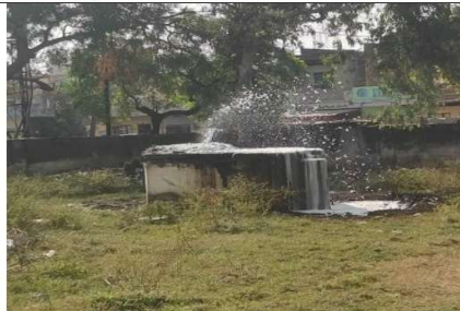
Excessive flow at discharge point jetting out from final discharge line
