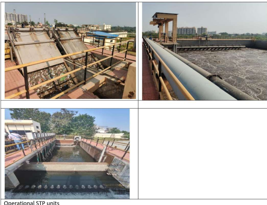
Operational STP units
