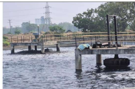
Aeration tank with defunct aerator.
