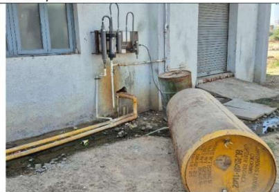
Chlorination system without any safety measures
