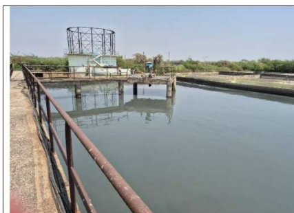
Aeration compartment without aerator
