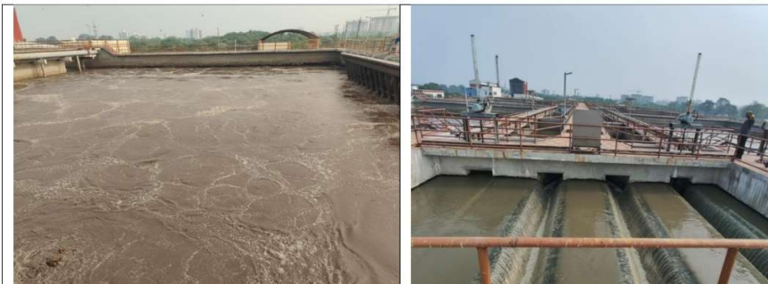
Operational units of STP.
