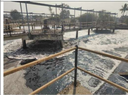
Black colored mixed liquor in aeration tank.
