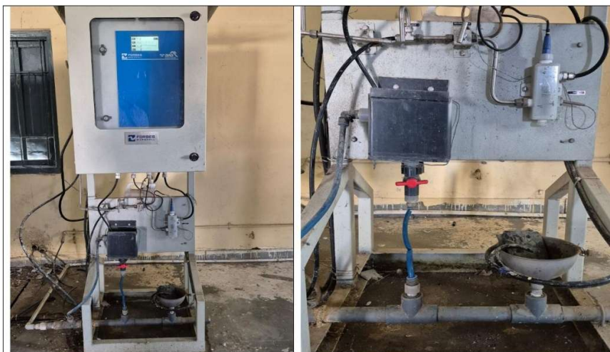
Defunct OCEMS showing misleading results of COD, TSS, BOD, and pH
