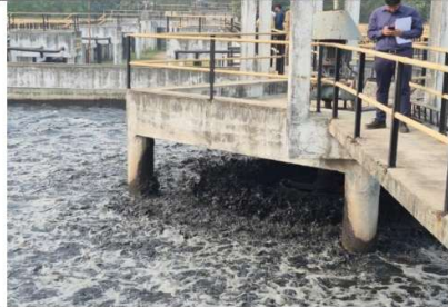
Black colored mixed liquor in aeration tank.
