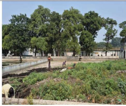
Sludge drying bed with vegetation.
