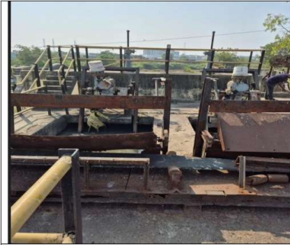
Completely corroded and non-functional screen chambers.
