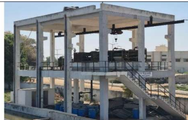
Sludge dewatering system not in operation
