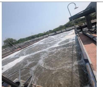
White foam in MBBR tank and lack of PVA gel media
