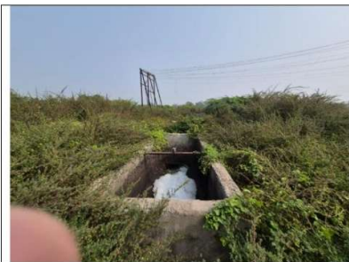
Parshall Flume covered with foam.
