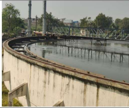
Primary clarifier mechanism out of order since 2017.
