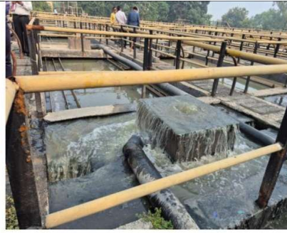
Division boxes on UASB were found overflowing
