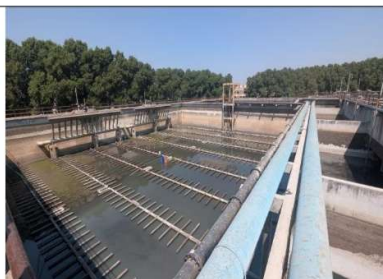
SBR under maintainance
