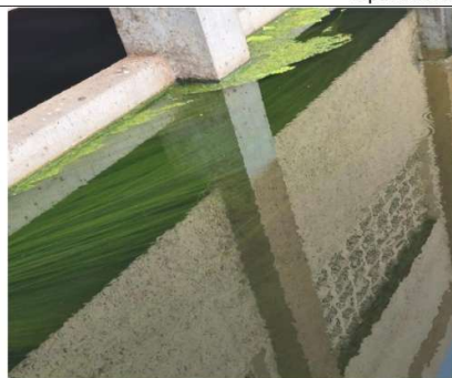
Growth of algae in chlorination tank
