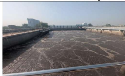
SBR in aeration mode
