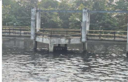
Aeration tank with defunct aerator
